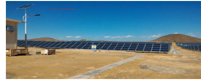
Figure 12 Global view of a part of the PV plant of Oued-Kebrit (Algeria)
